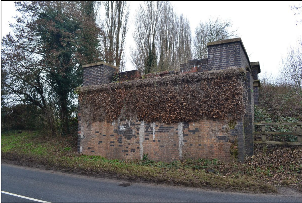
Photograph 41: View west towards the former eastern support of the railway bridge over Gainsborough Road, at the eastern extent of the Grade II* Listed Torksey Viaduct (NHLE 1359456).
